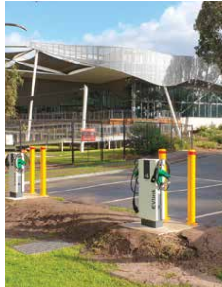
The new electric vehicle charging stations.
